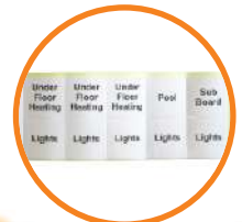
Label Circuits Clearly and Neatly for Easy Identification
